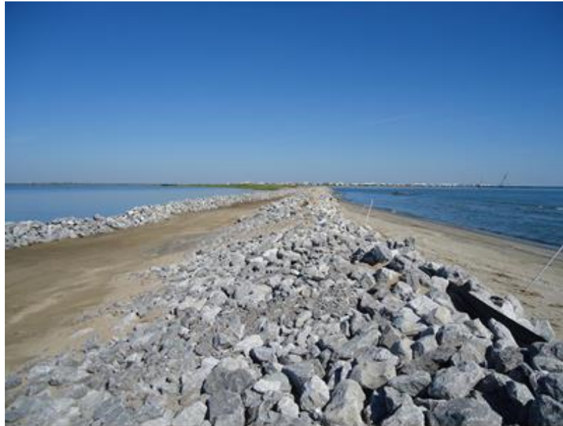
Figure 2 Repair of breach at Caminada Pass using rocks and sand; location indicated on Figure 1 (Berm created by LAANG, 2010)
